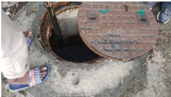
Fig. 5 Checking consistency of sewage in settling tank
