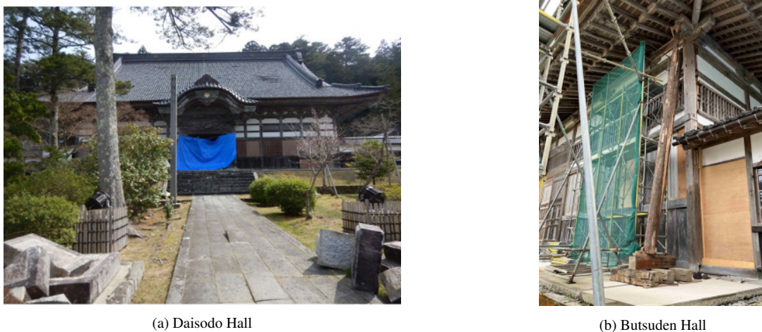
Figure 9: Damage to halls in Soujiji Soin Temple
