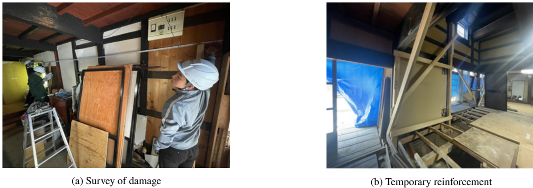
Figure 16: Emergency response work at Wajima Kuroshima Preservation District of Groups of Traditional Buildings
