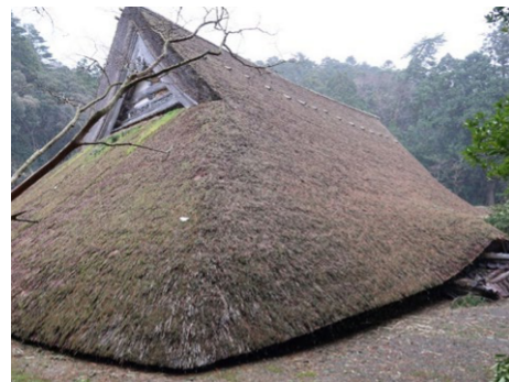
(b) After Earthquake
