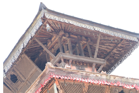
Figure 1. Damaged state after the 2016 Gorkha earthquake
