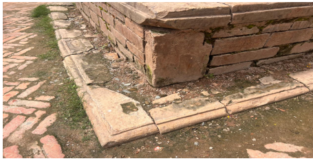
Figure 8. Misplacement of overall superstructure over plinth
