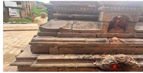
Figure 9. Misplacement of elements during reconstruction
