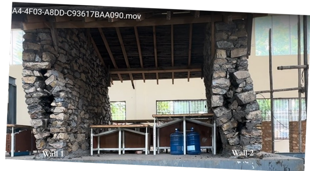
Figure 12. Contact of desks A and B with Wall 2 temporarily stabilizes wall interior wall wythe of wall 2. portion of wall 2 NOT in contact buckles.
