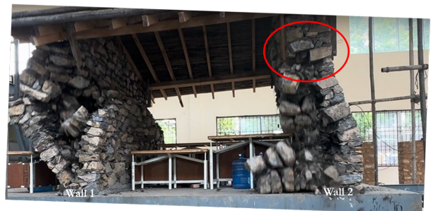
Figure 13. Wall 1 wythes buckle in opposite direction. Wall 1 loses load bearing capacity. Roof begins to fall. Roof-wall connections hold wall 2 together (somewhat).
