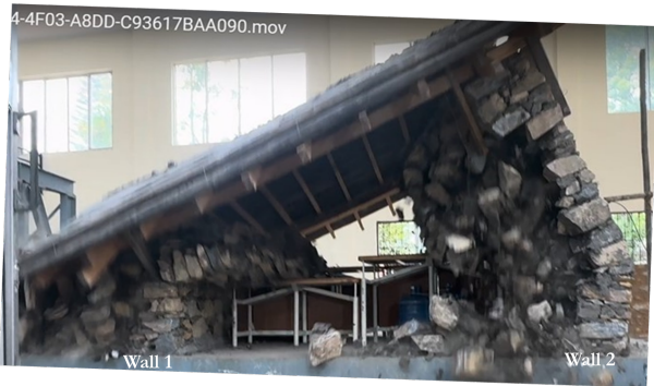
Figure 14. Roof over wall 1 collapses. wall 2 loses load bearing capacity.
