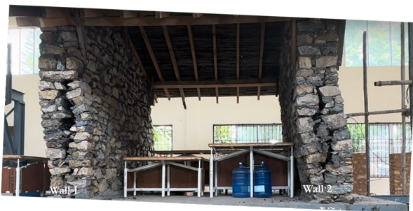
Figure 11. Second pendulum impact (Shock #7) produces additional shear in the walls and further separates wall wythes.
