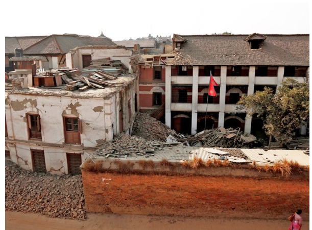
Figure 6. Building damaged by earthquake
