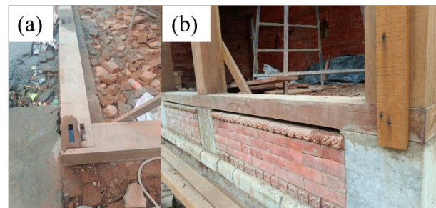
Figure 4. Timber joint (a) Groove in plinth tie for post connection (b) Plint tie beam to post connection
