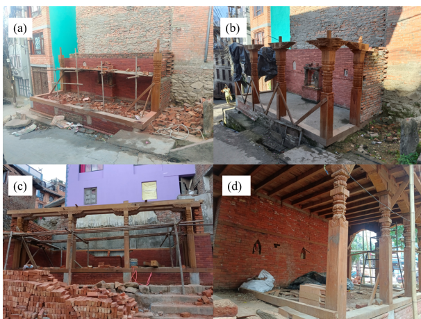
Figure 3. The construction sequence of rest house in Kirtipur. (a) Construction completion of plinth tie and partial completion of side wall., (b) Erection completion of post with corbel, (c) Construction completion of the floor beam and (d) construction of floor joist
