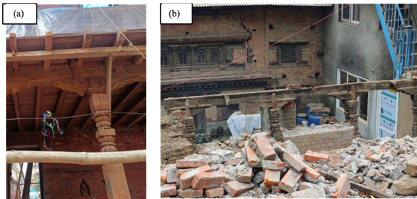
Figure 6. Timber joints (a) Beam post connection using bracket (b) Post dowel end observed in old demolished building
