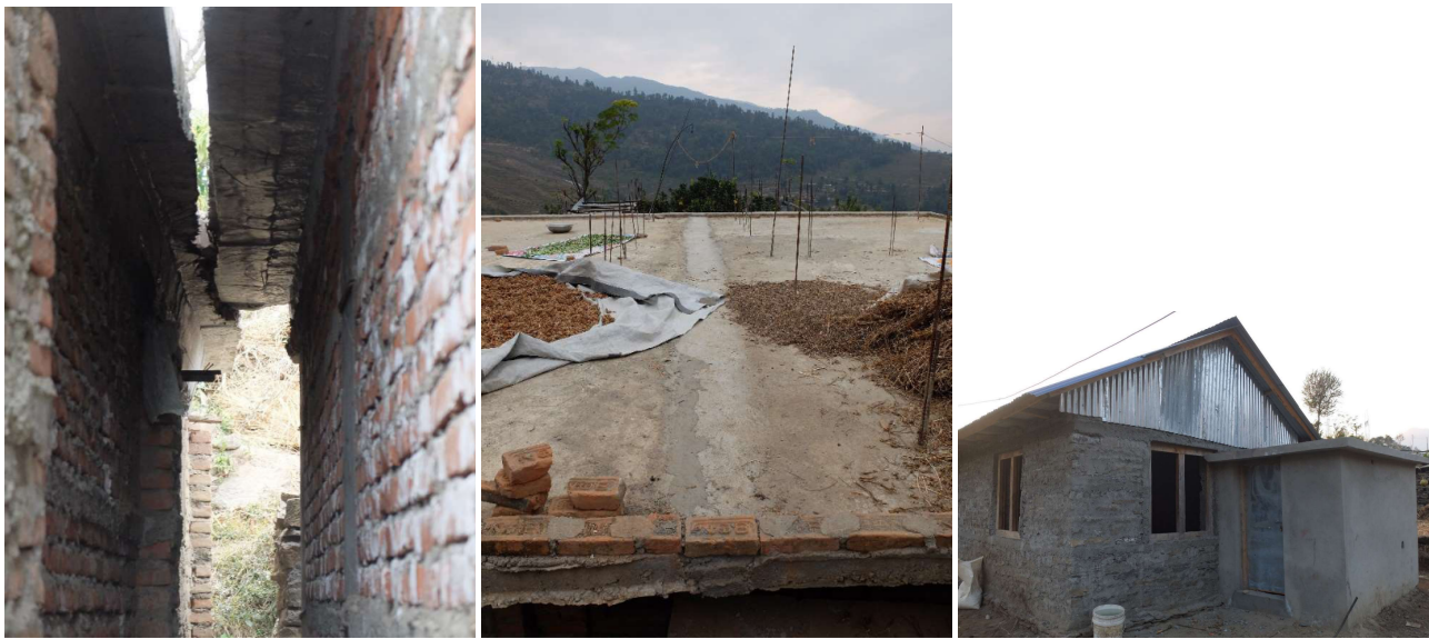
(a) Two dwellings merged without an appropriate technical solution (b) Reinforcing bars exposed to corrosion for future vertical extension (c) Risk of damage to the newly built house unit due to the addition of toilet without recommended gap/technical solution
