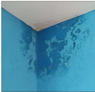
Figure 10: Seepage inside rooms due to poor construction quality
