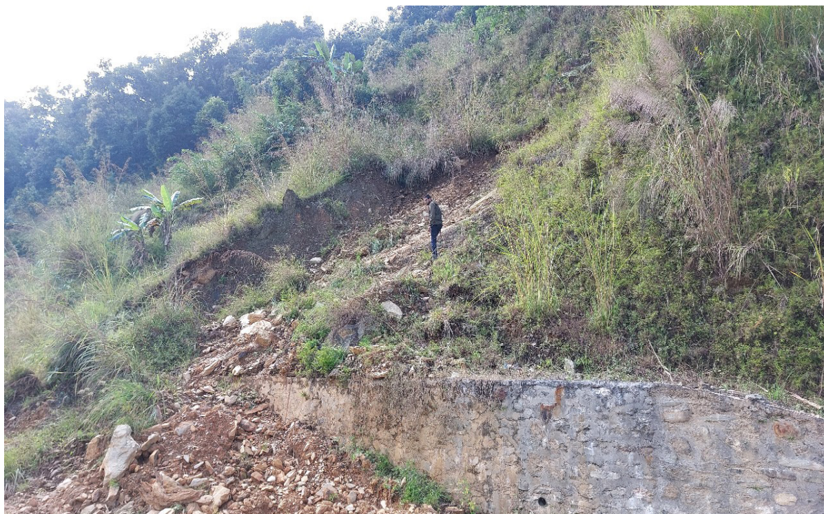
Fig. 2: Landslide observed along the Pokhara-Syangja road section
