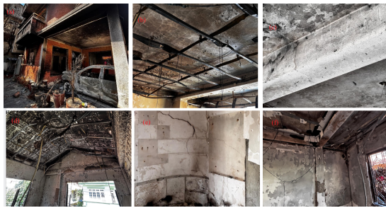
Figure 8: Showing damages in various locations of Building C (a) Exterior view of an RCC building showing fire damage (b) Fire-affected RCC slab soffit with extensive soot accumulation and exposed suspended service lines, indicating prolonged fire duration and elevated ceiling temperatures (c) Close-up view of an RCC beam exhibiting surface discoloration, fine flexural cracking, and localized material degradation due to elevated temperature exposure (d) Damage to slab–beam junction with partial loss of plaster cover, exposed reinforcement, and hanging electrical conduits following intense fire action (e) Interior wall and column surface showing cracking, plaster debonding, and thermal discoloration (f) Beam–column joint with plaster spalling, cracking, and exposed reinforcement, highlighting degradation of load-critical regions under fire exposure
