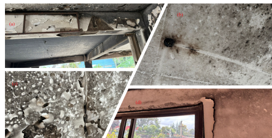
Figure 6: Showing damages in various locations of Building A (a) Fire-damaged structural beam showing extensive soot deposition, blistered paint, and heat-induced surface cracking (b) Damage in electrical point and crack propagated in slab along the line of wiring (c) Porous, bubbled surface texture—classic signs of thermal decomposition of cement paste due to high fire temperatures (d) Fire-induced spalling of concrete
