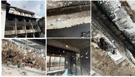
Figure 7: Showing damages in various locations of Building B (a) Discoloration of outer face of building due to fire (b) Fire-induced spalling of concrete with exposed reinforcement in the beam soffit (circled in red) (c) Porous, bubbled surface texture-classic signs of thermal decomposition of cement paste due to high fire temperatures (d) Fire-damaged structural beam showing extensive soot deposition, blistered paint, and heat-induced surface cracking (e) Damage in electrical point
