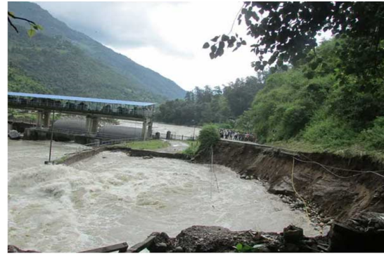
Figure 1: The Jure landslide (2014) damaged the road and headwork of the Sunkoshi hydropower project [17]
