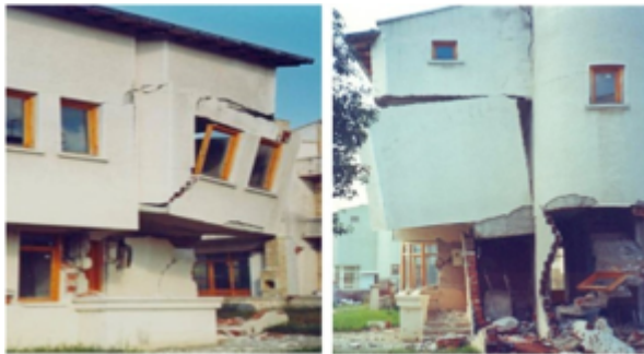
Figure 1: Damage of Structure Overhangs during 1999 Turkey Earthquake[4]
