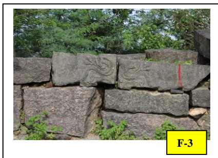
Fig-3 is that of the inner ring in the afar – SE side - of the impact created water hole. There is disorder in the stack. The etching suggests possible stacking during conservation & site clean exercise. Fig-4 is that of the also of the same wall (battlement) at the front gate. Fig-5 indicates the large width dimension of the earth\rubble outer ring\battlement; East. Photo –own.
