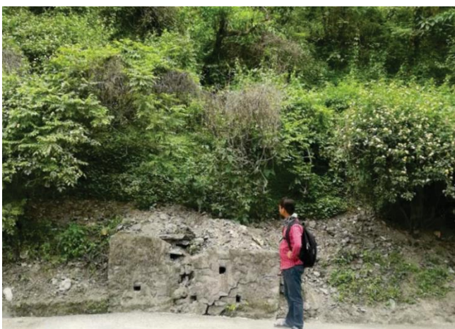
Fig. 7: Development of the tension crack destroys the wall installed for slope stabilization along the Koshi Highway
