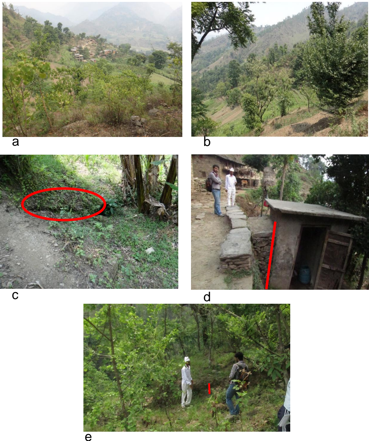
Figure 6: Several field features of the Kuyadaha landslide (a) and (b) Crown and body of landslide area (c) crack developed near crown (d) tilted toilet and (e) displacement of the landslide
