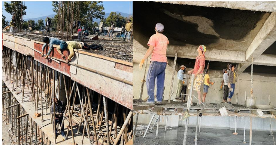
Figure 2: Lack of Safety equipment (Helmet, Harness, Glasses, and Gloves) during construction work
