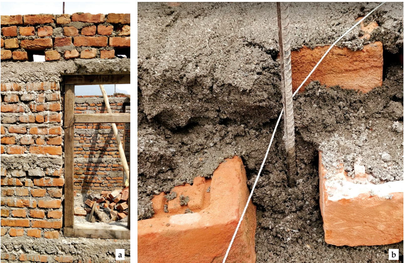
Figure 32: (a) Jamb rebar exposed on window side (b) rebar embedded in concrete wall in mortar
