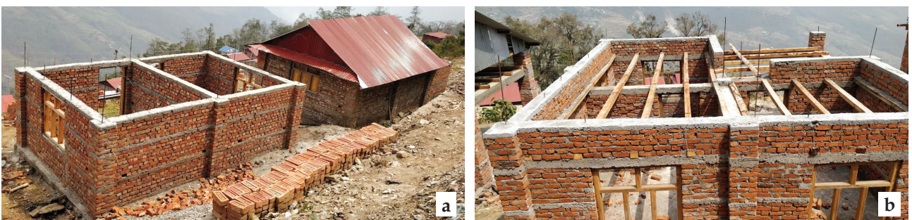
Figure 16. (a) Constructed wall in the buildings (b) Some vertical rebar terminated with insufficient development length.
