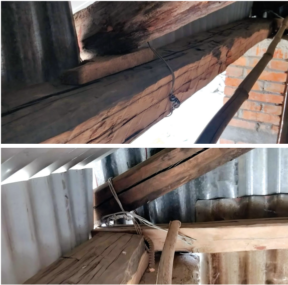
Figure 22. GI wire used to tie the rafter with timber band at eaves and with vertical rebar.
