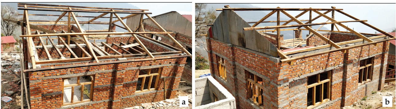
Figure 21. (a) Roofing structure and floor joists. Rafters are anchored by bending the vertical rebar around it. (b) Fixing appropriately cut gable sheet before fixing roofing sheet.
