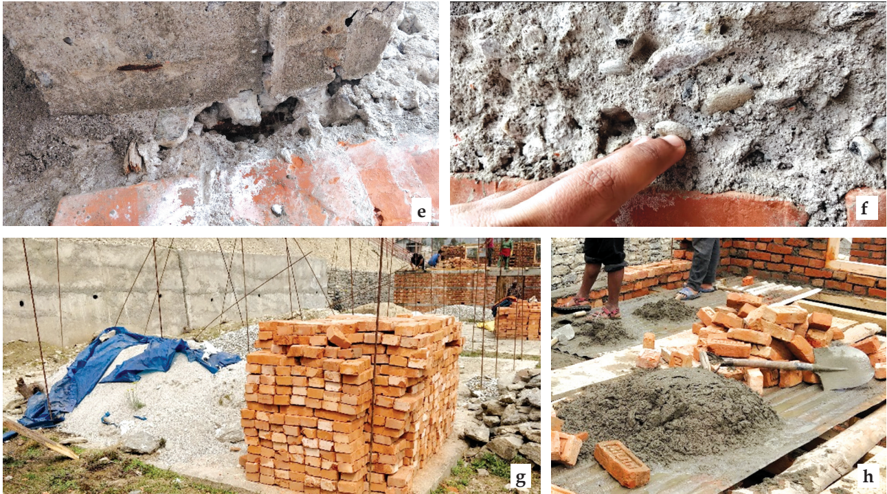
Figure 29. Various concrete defects in reconstructed houses (a-e) honeycombing and exposure of rebar in bands (f) very poor-quality powdery concrete easily scratchable by hand, (g) sand stockpiling with vegetation (h) prepared mortar for construction.
