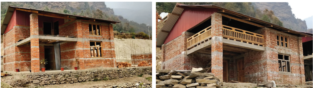
Figure 12. Two storey construction with missing dowel band in first floor
