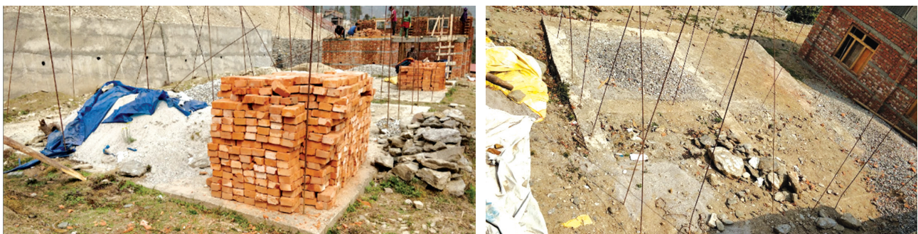
Figure 30: Vertical rebar left unprotected at plinth
