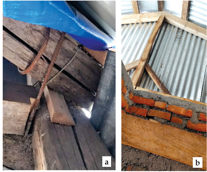
Figure 23. (a) Tying of rafter with vertical rebar (b) Tying of rafter with GI wire from eaves band, bracing of vertical post of roofing structure.
