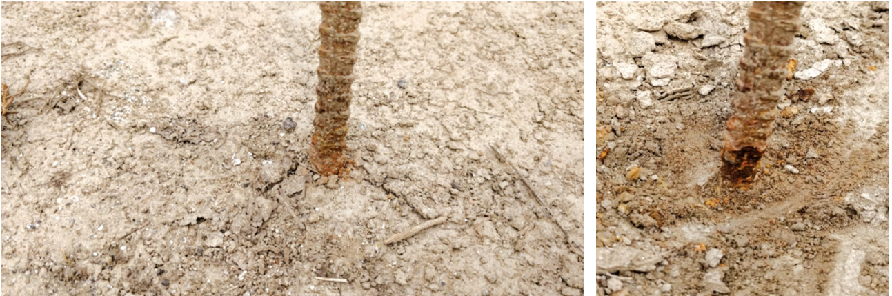
Figure 31: Corrosion of vertical rebar near plinth
