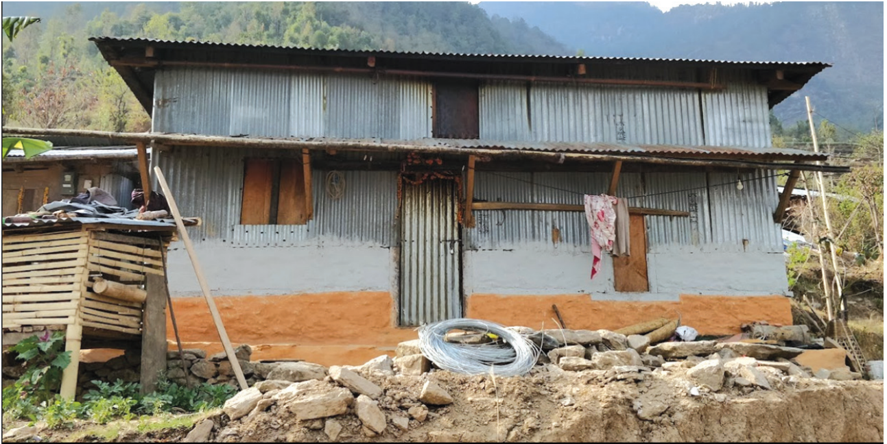
Figure 2. Half height of old building was retained to rebuild CGI sheeted two-storey building.
