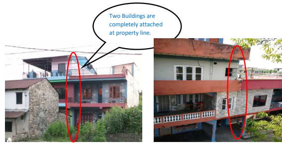
Figure 1 Common Construction Practice in Pokhara Metropolitan City/Problem in Construction Practice
