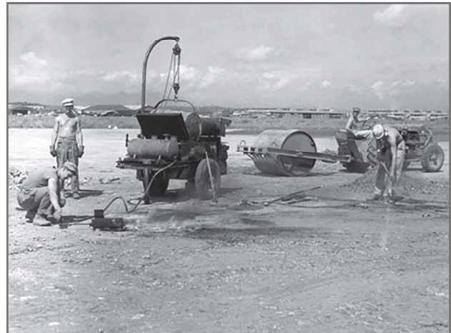
The 872d Airborne Engineers repair the runway on Atsugi Airrome, Japan. The asphalt "kettle" was used to liquefy barrels of asphalt that was spread over areas under repair, 1945.
