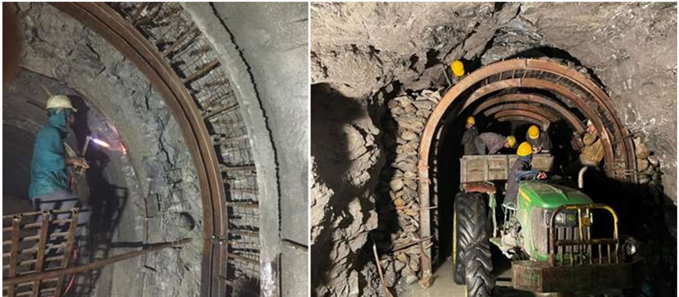
Fig. 10: Practiced support system in fracture rock mass in Nepal. Left: A worker is busy welding the reinforcement bars to connect with applied steel ribs. Right: The workers are stone packing behind bars.
