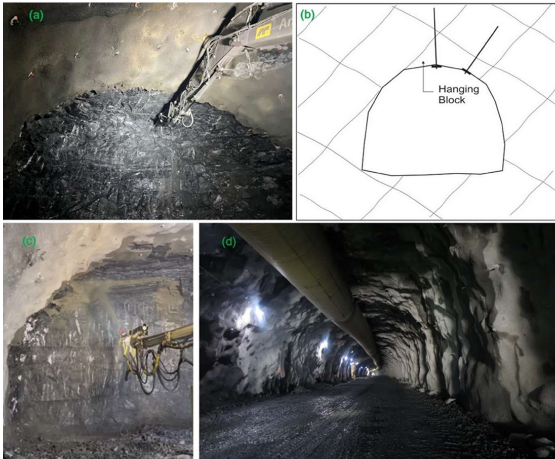
Fig. 5: Application of rock support in NMT; a) Mechanical scaling, b) Spot bolting to hold loosened rock block, c) Application of steel fiber shotcrete and d) A tunnel reinforced with the application of systematic bolting and steel fiber shotcrete as final rock support.
