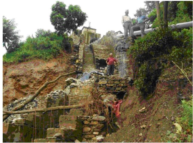
Fig. 1: Slope failure just down the forebay of the Mardi Khola small hydropower project (3 MW) (July 2010)
