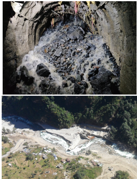
Fig. 1: Tunnel collapse and water ingress of Khani khola hydro project and Bhote Koshi dam damaged by GLOF in 2016.
