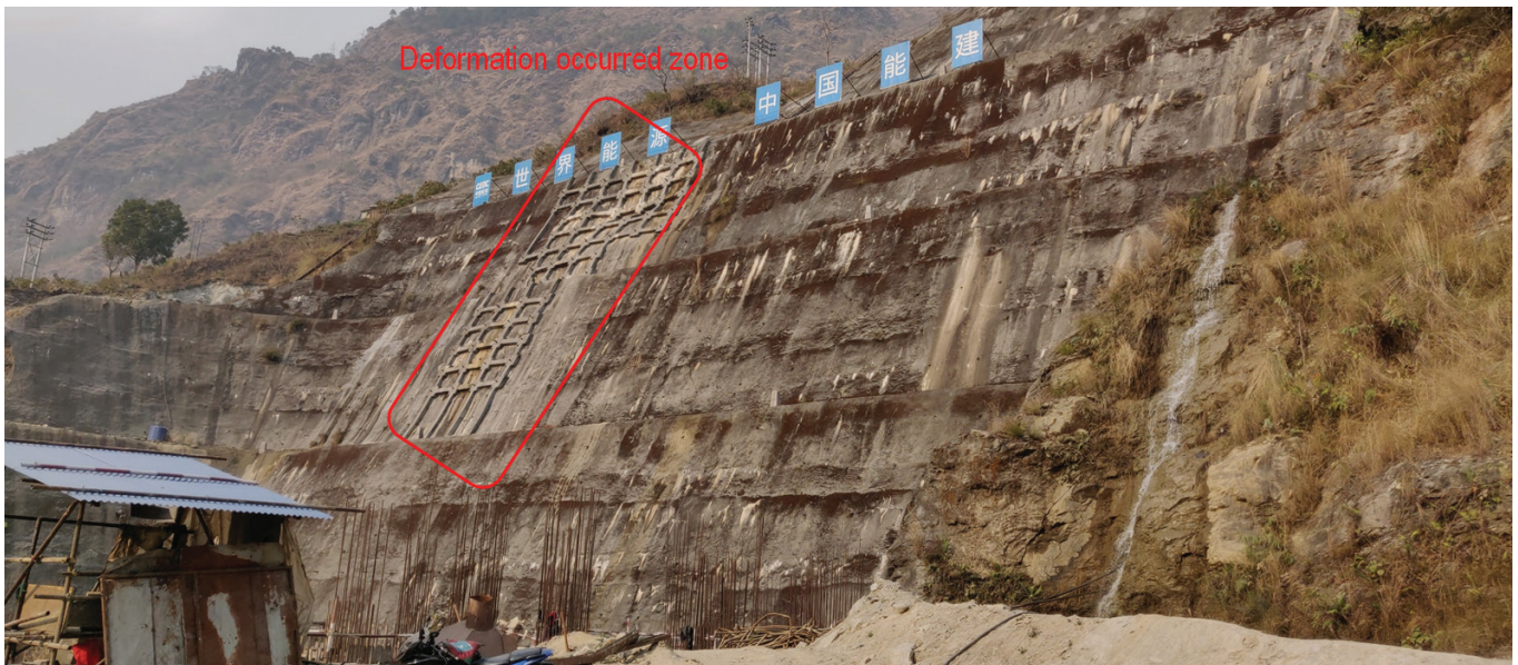
Fig. 2: Deformation area in cut-slope and secondary support application.
