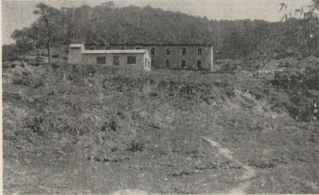
Figure 5: Figures showing subsidence of ground surface at College Hostel (Dhankuta Bazar).
