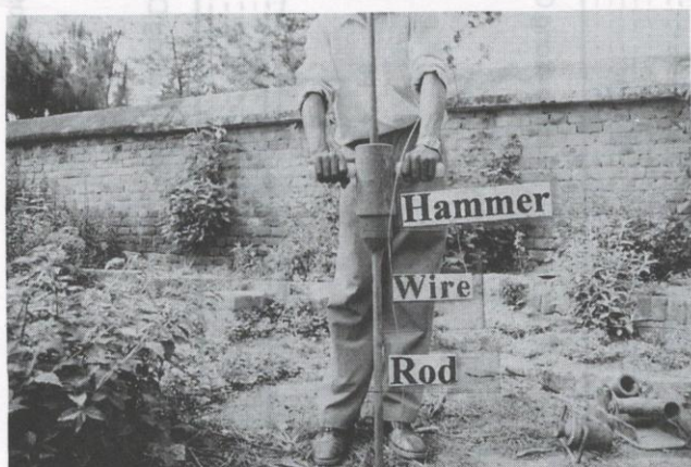
Plate 1a: Installation of RDT and VWE
