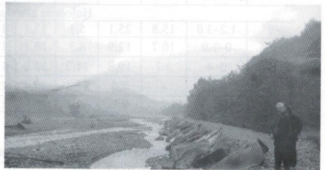
Fig. 13: Right bank of Gizeldon River about 1 km below Genaldon River mouth (Ph1 in Fig. 11). The road was washed away by an ordinary summer flood (10 m 3 /sec). Photo by E. Zaporozhchenko, 1 June 2004
