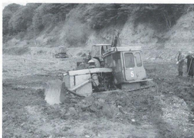
Fig. 10: Right bank of Gizeldon River about 1 km down the Genaldon River mouth. The road was washed away by an ordinary summer flood of 10 \text{ m}^3/\text{sec} . Photo by E. Zaporozhchenko, 1 June 2004
