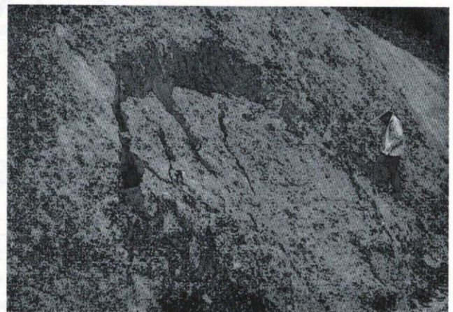
Fig. 14: Close-up view of wedge failure on sheared mudstone and fractured sandstone at Km 49
