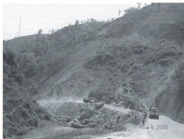
Fig. 7: Dolalghat Landslide which destroyed Arniko Highway on July 2003
