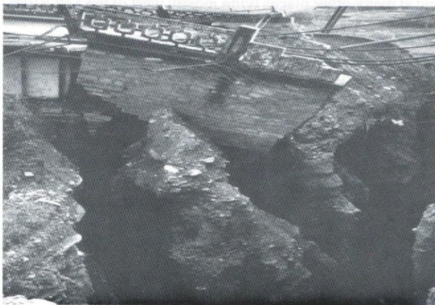
Fig. 6: Collapsed highway bridge over the Seti River at Pokhara
