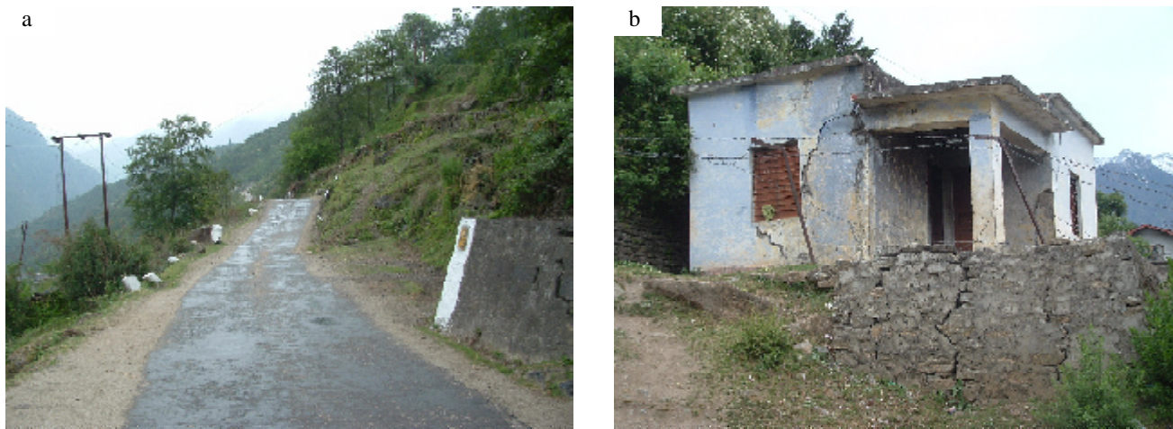
Fig. 2a: Road sinking due to a large rotational slide at Oucha, view to W; Fig. 2b: A cracked house due to ground subsidence at Joshimath
