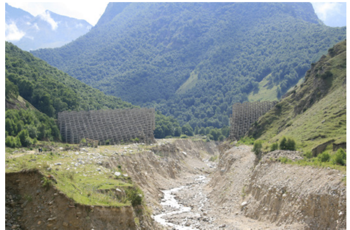
Fig. 2: A structure built for protection of the town of Tyrnyauz on the Gerkhozhan-Suu River was destroyed by a debris flow in 1999.
