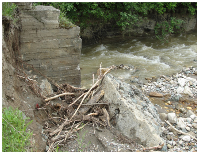
Fig. 9: Washout of the upstream slope and destruction of a part of a reinforced concrete structure of the entry portal of the tunnel on the Gizhgut River as a result of a debris flow of May 21, 2014.
