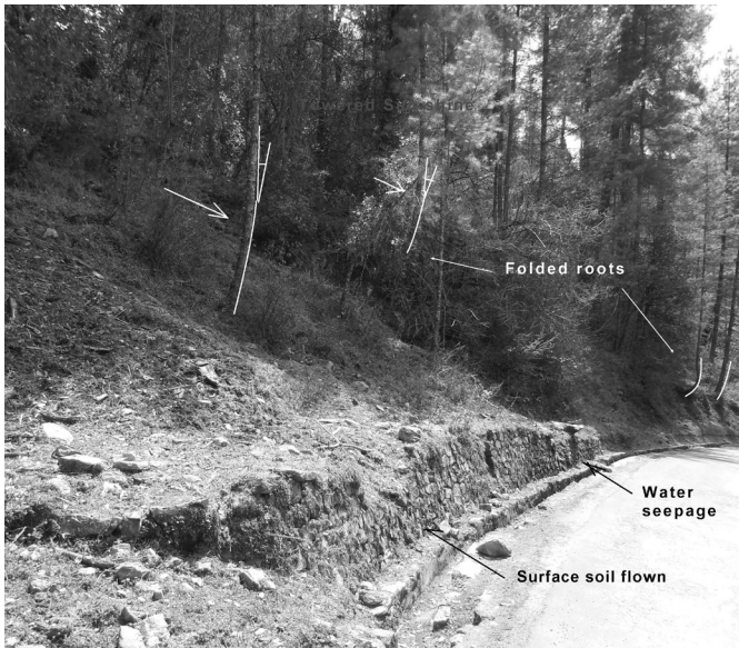
Fig. 14: Phenomenon of landslide in ‘No. a’ (roots bent, water seepage, surface soil flow).
