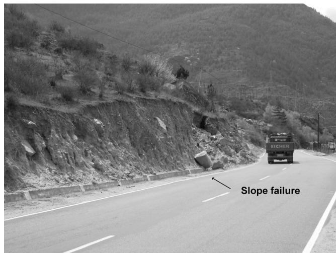
Fig. 20: The slope failure of the road cutting in ‘No. d’.
