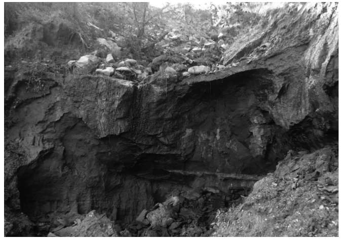
Fig. 9: Seepage and erosion observed at left bank of the Dhobi Khola near Budhanilkantha
