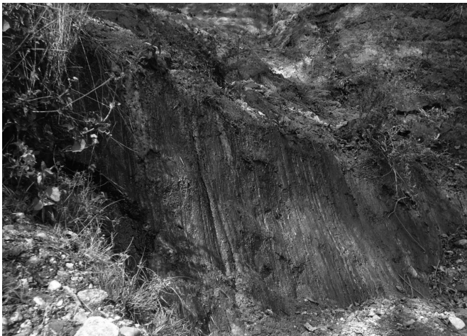
Fig. 8: Piping erosion observed at left bank of the Bishnumati River near Dhapasi
