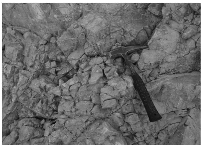
Fig. 7: Pink-Bitule Dolomite at the newly constructed damsite, on the right bank of the Chameliya River, Darchula
