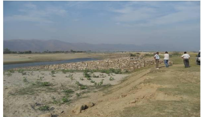
Figure 10: Spur with inclined crest (Narayani River)
