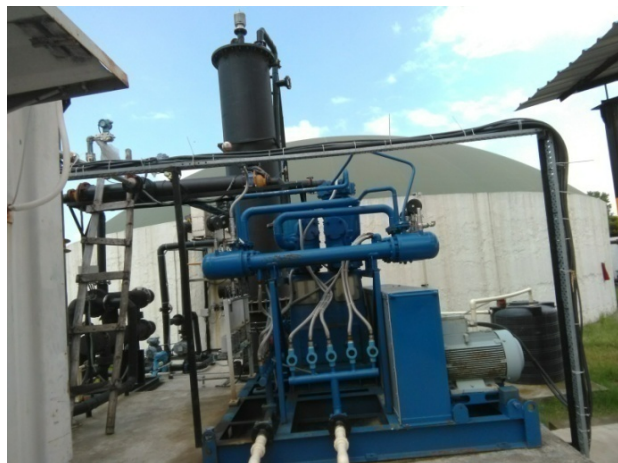
Figure 5: Digester and H_2S scrubber
