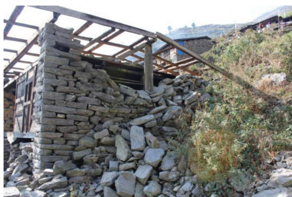
Fig. 5: A picture of a house in Haku where the dry-stone gable collapsed
