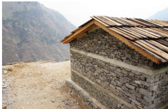
Fig. 6: New house built in Gatlang village with horizontal RCC banding and cement mortar
