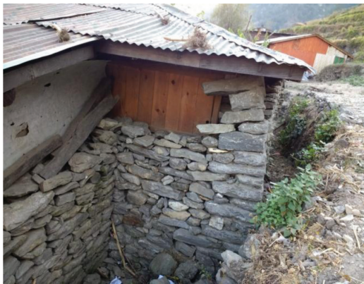
Fig. 2: Corners of wall collapsed due to lacking mortar and horizontal banding
