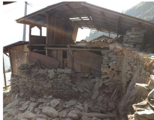
Fig. 3: A house in Haku which kept the roof from collapsing due to its wooden structure of the front wall, floors and buried back wall
