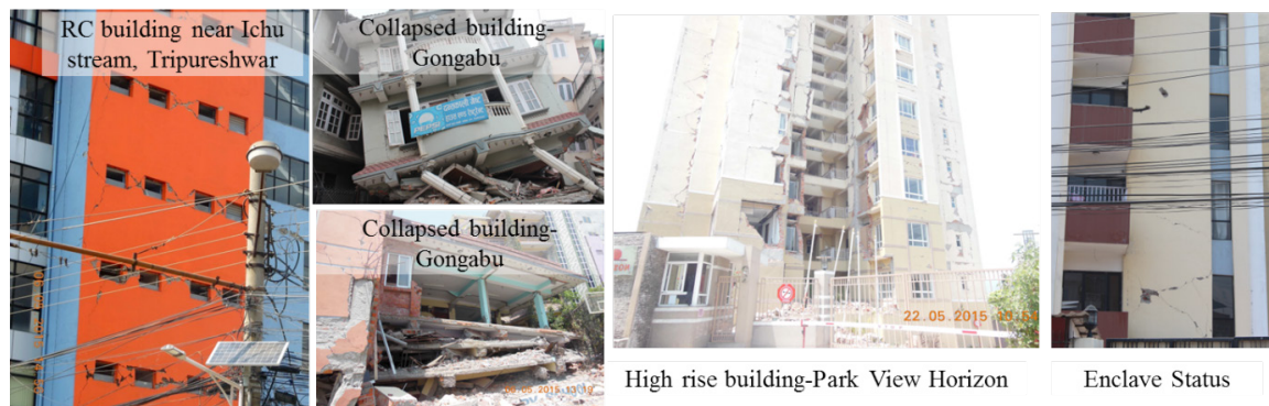
Fig. 14. Severely damaged well-designed buildings
