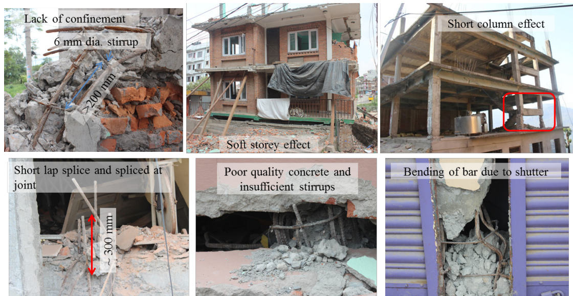
Fig. 4: Typical failures observed in RC buildings.
