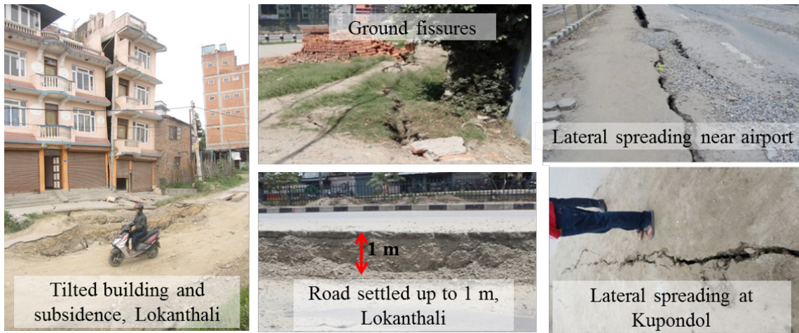
Fig. 12: Typical lateral spreading and settlement caused by the earthquake
