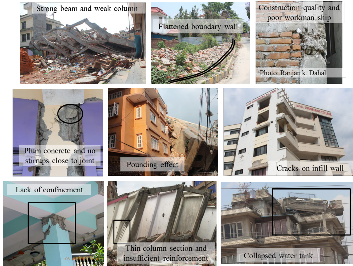
Fig. 5: Typical failure observed in RC building during the reconnaissance.
