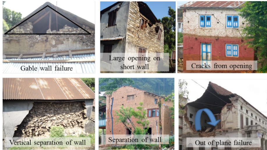
Fig. 6: Typical failures observed in masonry buildings.
