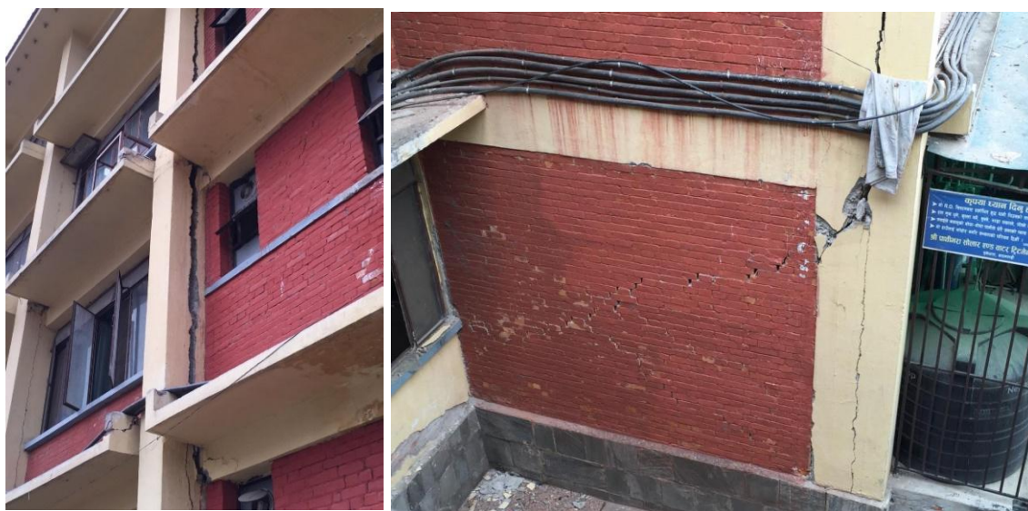
Fig. 11: Failure of Column Joints during April 2015 Earthquake (Source : EERI) [7]
