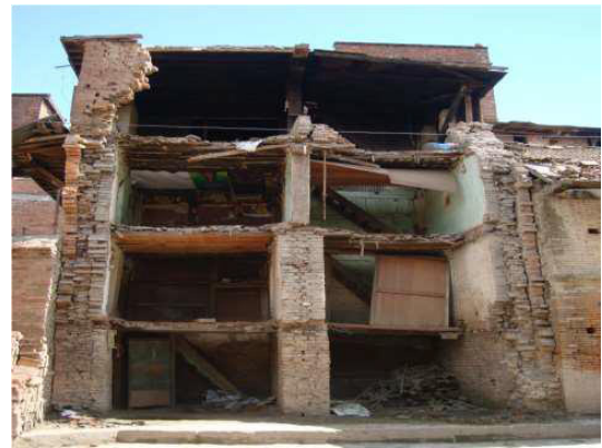
(b) Out of plane failure [15]
