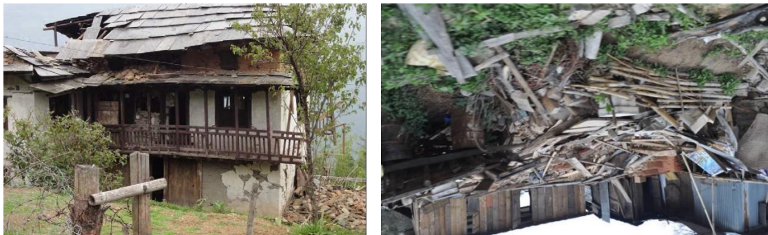
Fig. 10: Wooden buildings after Earthquake on 25 th April 2015 (Source: EERI) [7]
