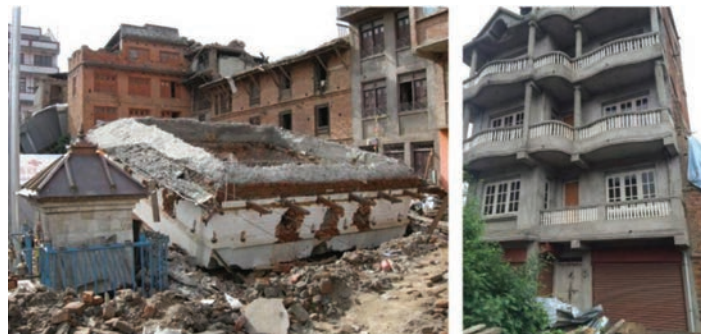
Fig. 10: Pancake failure of a Sankhu temple (Left), soft storey on ground floor in a tall building in Sankhu (right)
