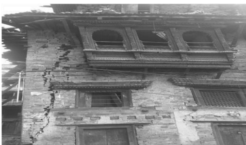
Fig.23: Tension failure of building.
