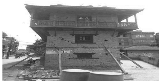
Fig.22: Shear failure of building.
