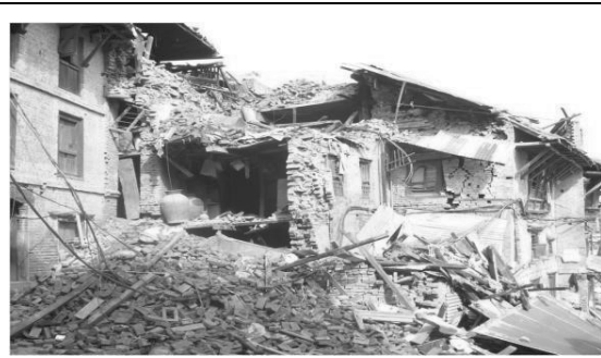
Fig. 28: Mixed failure mode of building.
