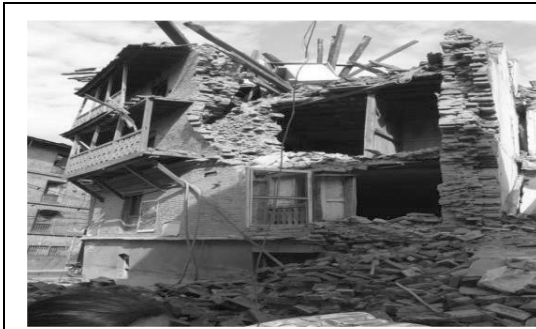
Fig. 27: Torsion failure of building.
