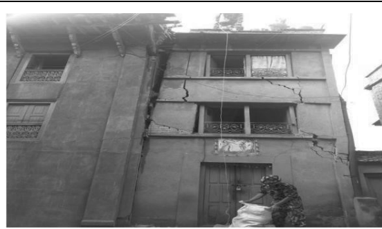
Fig. 26: Pounding effect between two buildings.
