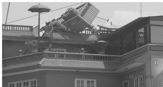
Fig. 18: Water tank collapse.
