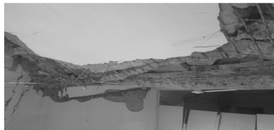
Fig. 16: Flexural failure of slab.
