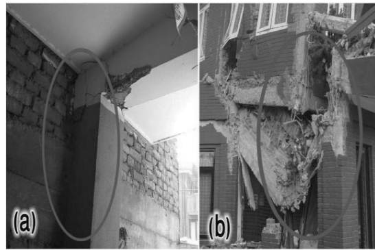
Fig. 14: Beam–column joint failure: (a) shear failure; and (b) brittle failure.
