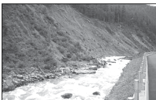
Figure 16: Road construction push the river other side erode the toe of the slope increasing slope failure
