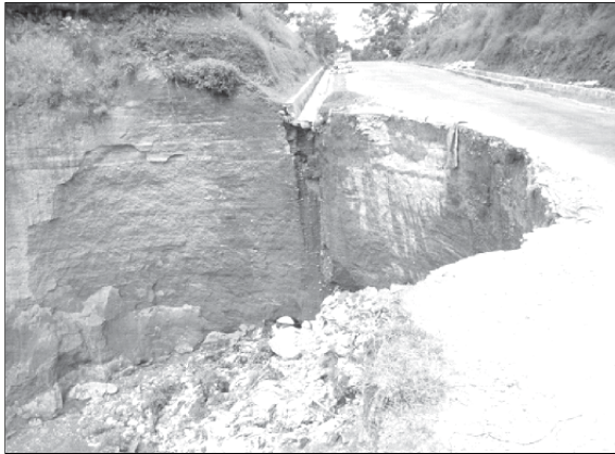
Figure 2: Concentrating drainage from larger distance causing erosion. Kathmandu- Pokhara Highway, Tanahu district
