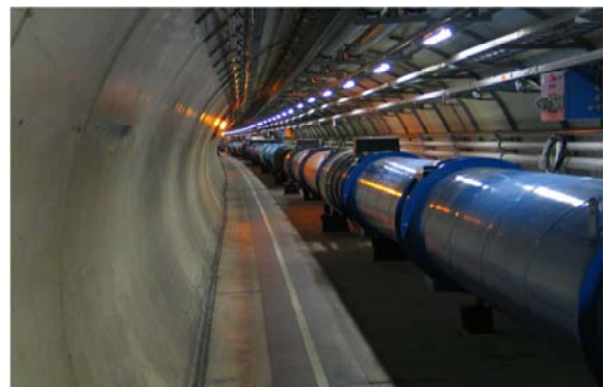
Fig 6 . The superconducting magnets in the LHC tunnel
