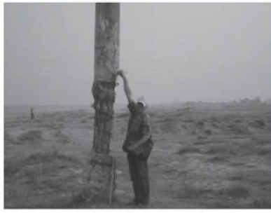
Figure 8. Electric pole hanging
