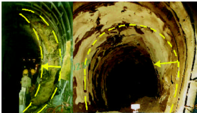
Figure 8. Severe squeezing at Modi pressure tunnel (left) and Kali Gandaki headrace tunnel (right) (Photo: Himat Hydro 2001 and Impregilo SpA 1989)
