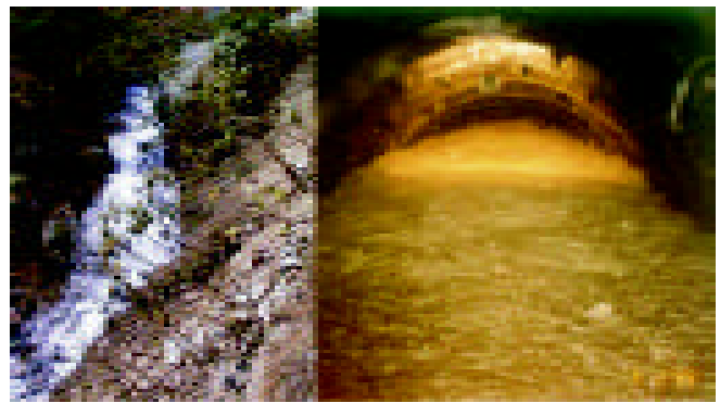
Figure 9. Water leakage from adit 2 of Khimti headrace tunnel after early water filling (left) and mass inflow of water mixed with debris from a shear fault at the pressure tunnel of Modi Khola (right) (right photo: Himat Hydro 1998)
