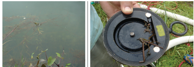
Figure 7. Dense Weed Growth in Peaking Pond and Debris Catching on the Valve Plate.
