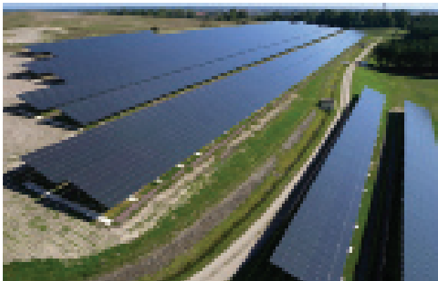
1.1 MW Nano Solar System in Germany
