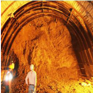
Figure 5. Showing shattered rock mass due to presence of many shear zones and damp to dripping water condition just after excavation in TRTs.
