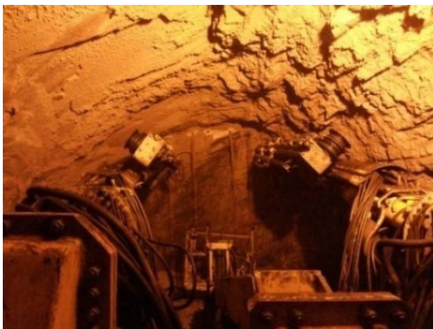
Figure 15. Photograph showing ingress of water from drainage holes drilled prior to face advancement
