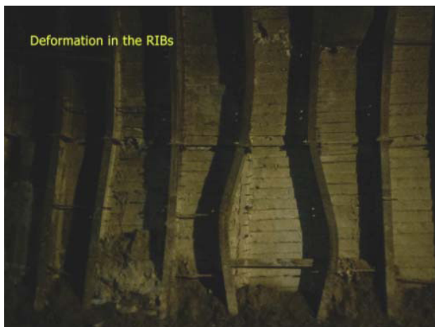
Figure 11. Photograph of buckled ribs in high
